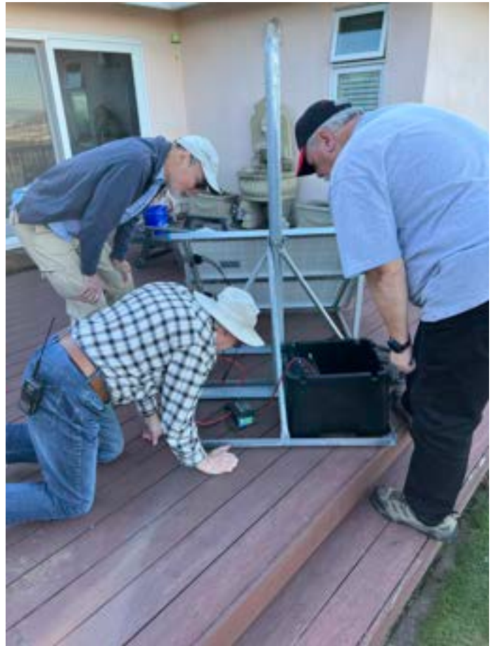
Constructing the 120 Sector Radio for the roof of Building 7 at Skyline College
